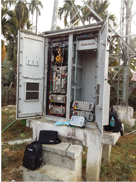
CellAdvisor tapping the BBU-RRH CPRI link — all measurements are at ground level
